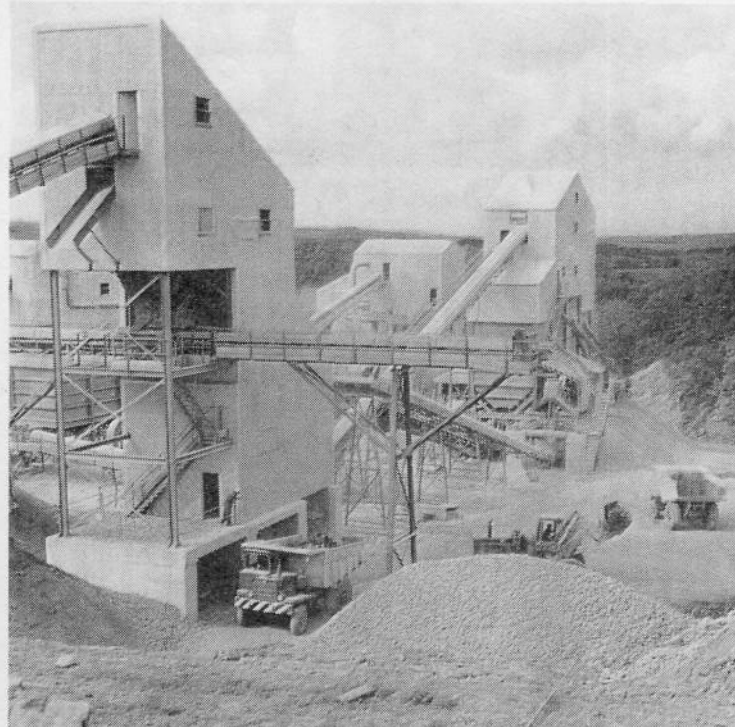
A quarry installation with Aveling-Barford Dumptrucks and Tractor Shovel in the foreground. The near building houses crushers and the far building taller screens and storage bins. Smaller of two far buildings is part of an asphalt plant working alongside the quarry plant.
