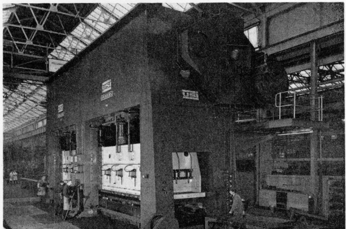
A general view of the new 4,000-ton chassis press installed by John Thompson Motor Pressings Ltd. Note the immense size of the plant when compared with men seen in the photograph.
