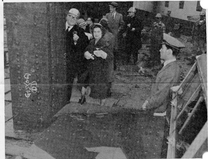
Shown locking-in first steel upright of the New York Hilton Hotel is Amy Vanderbilt, noted writer on social etiquette and cooking, with Eugene Voit, new hotel's general manager. Chauffeur-driven Land-Rover (foreground) was used to take VIP's and press photographers down steep muddy rainsoaked slope into pit.
