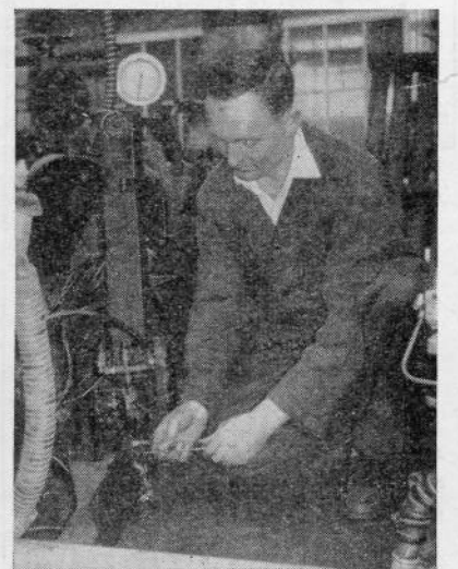
There is always plenty of work for the electricians during Operation Overhaul. Checking switchgear at Tyseley is Mr. D. Cockbill.
