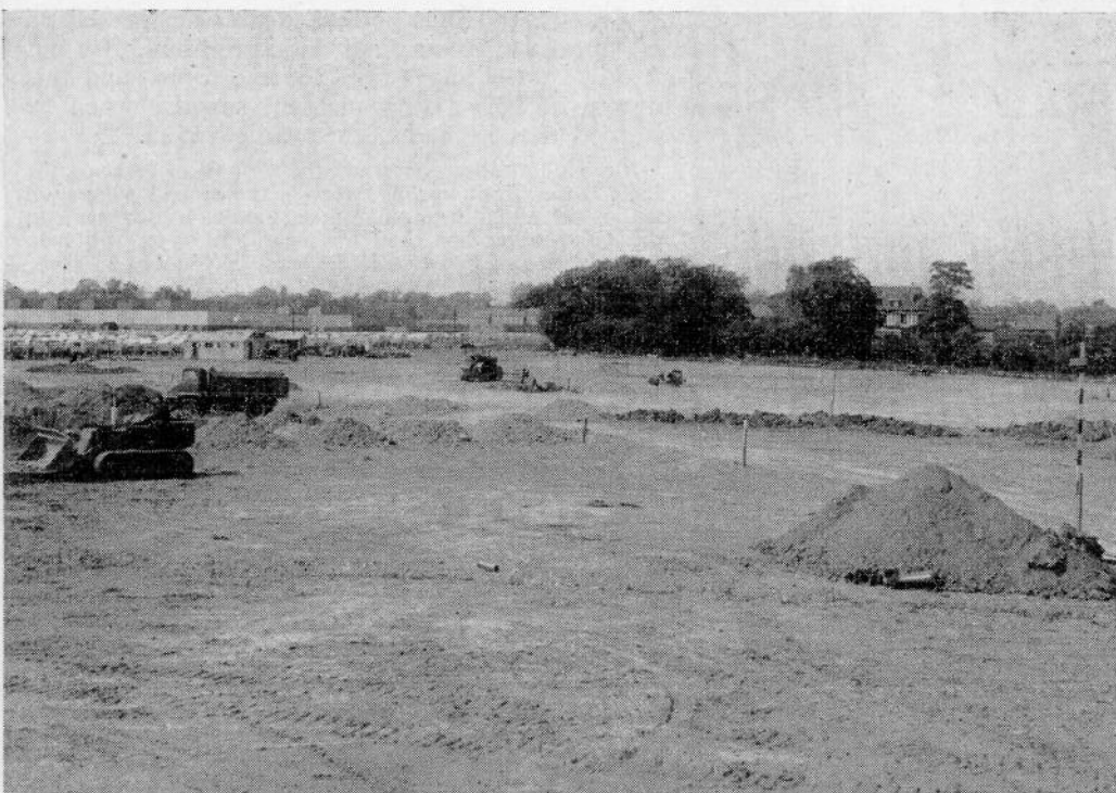
A photograph taken during the work on the North Site. The existing North Block buildings can be seen on the left of the picture.
