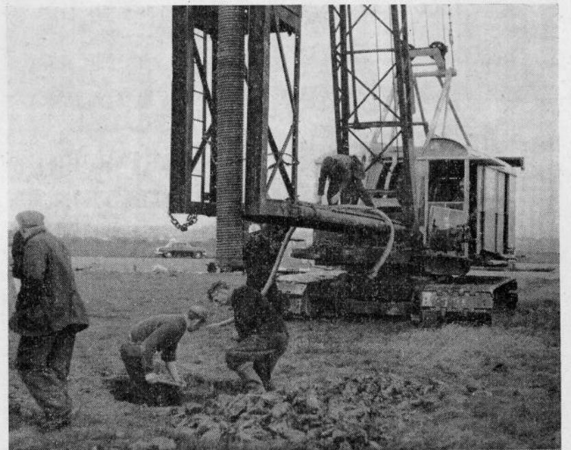
Pile-driving work in progress at Pengam Moors. Photo by courtesy of Western Mail and Echo Ltd.
